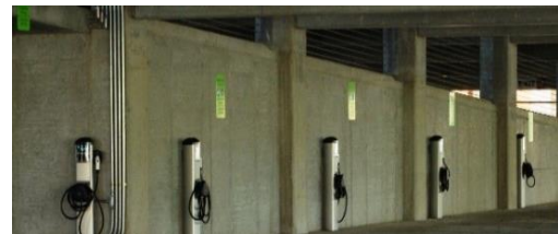
Electric vehicle charging spaces located within a parking structure.
